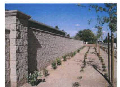
TAN COLORED SPLIT FACE CMU USED FOR SOUND WALL (ON CONCRETE RETAINING WHERE INDICATED)
