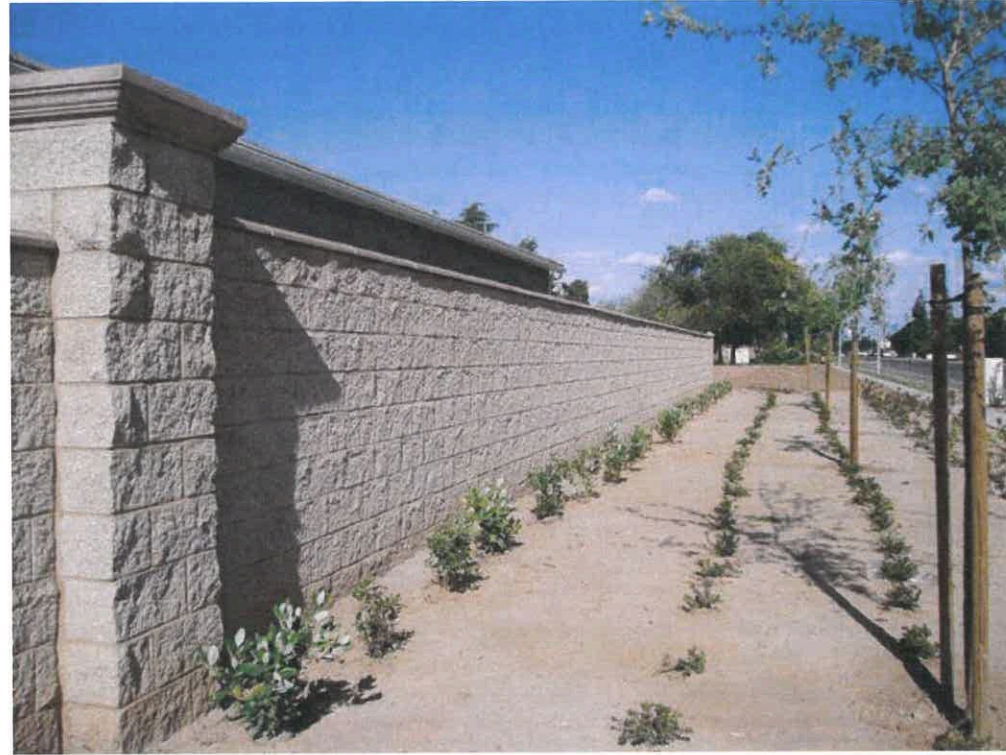
TAN COLORED SPLIT-FACE CMU (BOTH SIDES) WITH DECORATIVE CAP & DECORATIVE - CLAD PILASTERS WITH CAP SPACED AT A MINIMUM OF 40'-0" ON CONCRETE RETAINING WALL
